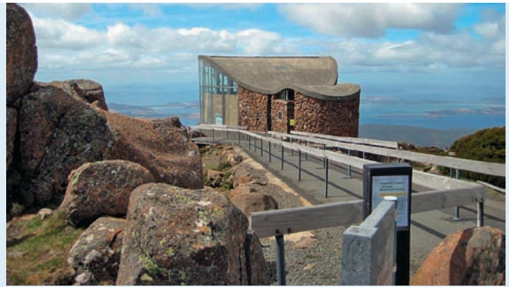
Hutchies has completed the internal refurbishment of Hobart's Pinnacle observation shelter at the summit of Mt Wellington.
