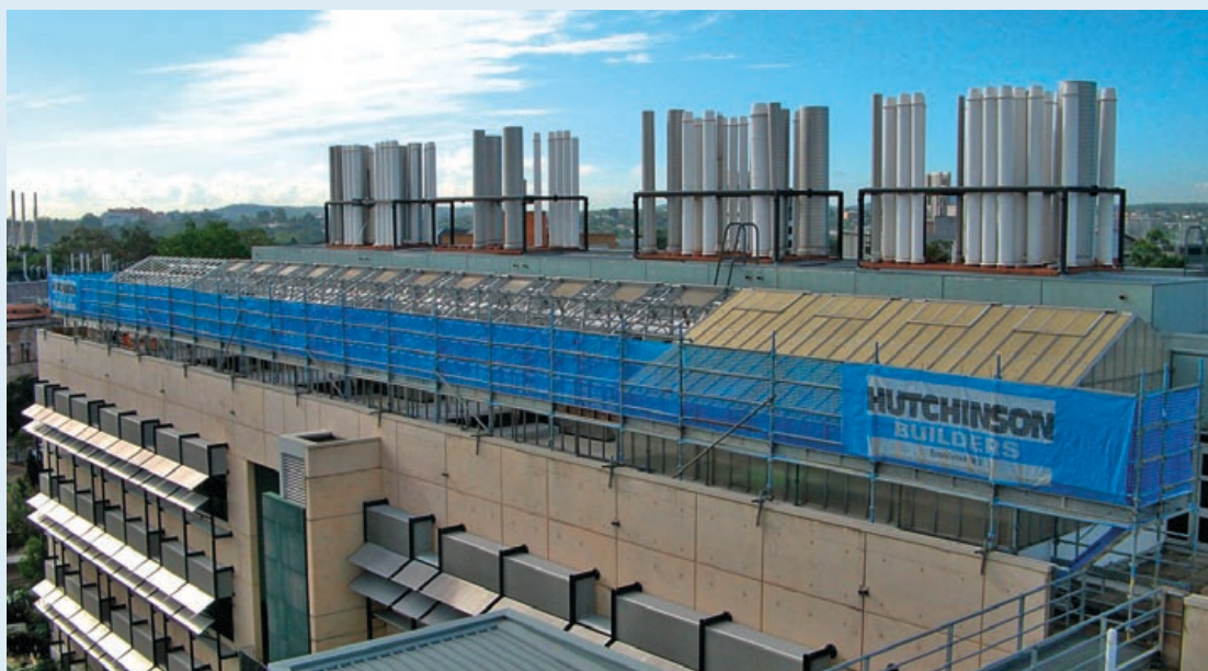
Hutchies is undertaking the expansion and refurbishment of CSIRO's rooftop glasshouses facilities on the University of Queensland campus.
